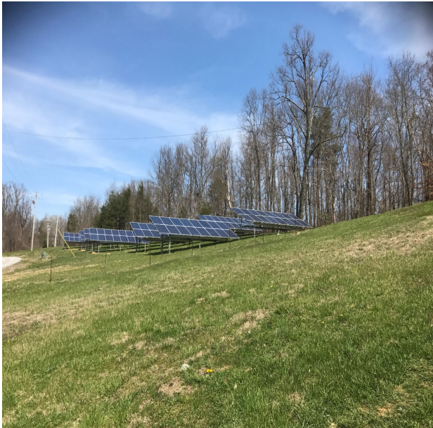
Monterey Water Plant Solar Array
